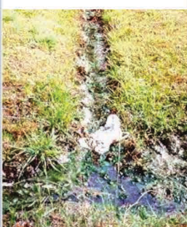
Failing Septic Systems
