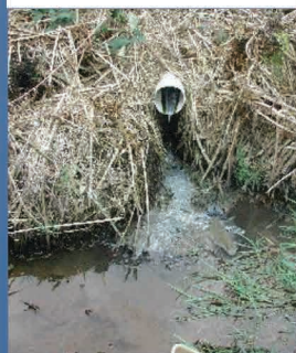
Illicit Sewer Discharges
