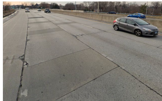
Exhibit 6: Worn pavement markings on this segment of I-95
